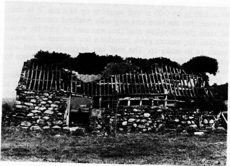
Fig. 2. The barn in process of dismantling: view of the crucks from the east
